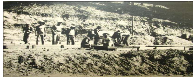
The late Rev. Dr. Bryan "Skipper" Hall works with a group to form footings for the building of Angie Smith Chapel at Sacramento. Hall is often remembered for his devotion to the Sacramento Methodist Assembly and its work camps for young people.
